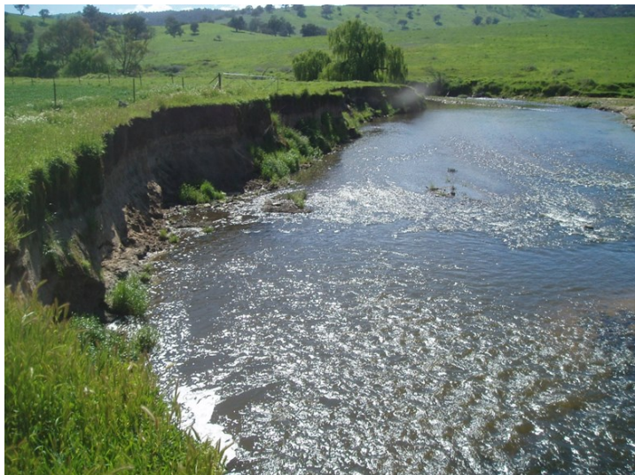
Before: Stream bank erosion from the 2012 flood event undercut a lucerne paddock on David Ham's property
