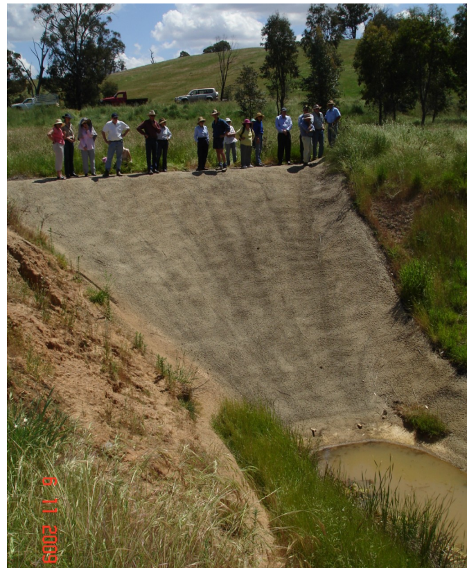
The Conways have been particularly impressed with the flume constructed to control erosion as part of a funded project, as it has stood up well to the recent severe rain events.
